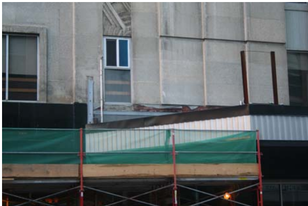
Photo 21 View of junction of limestone & black granite at left behind hoarding & scaffolding
