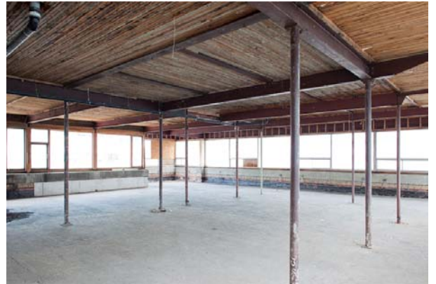
Photo 97 View of penthouse suite stripped down to bare structure w/ wood roof structural deck exposed
