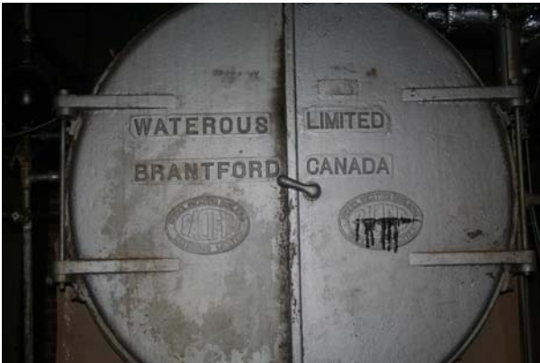
Photo 69 Detail view of boiler doors with manufacturer's name cast in the steel
