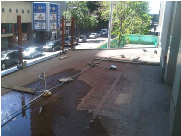
Photo 25 View of marquee roofing membrane, ponding water, & electrical conduit for lighting; 2 nd floor reinforced concrete slab cantilevers above front entry to form canopy for weather protection & marquee for Uptown Theatre
