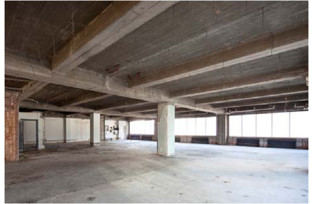
Photo 104 View looking NE toward exit door from west elevator lobby area on 4 th to 7 th floors, typical
