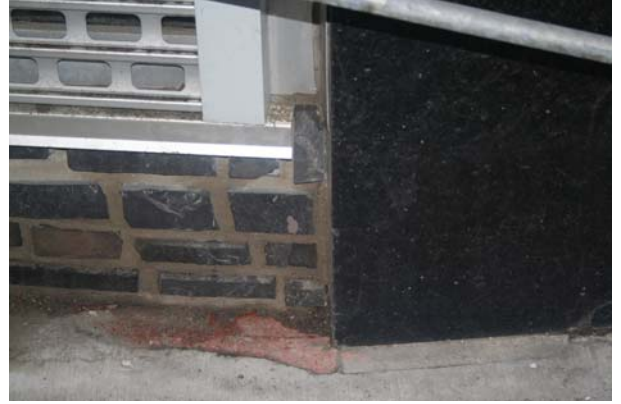
Photo 34 Detail view of Rundle rock to storefront grille to black granite juncture
