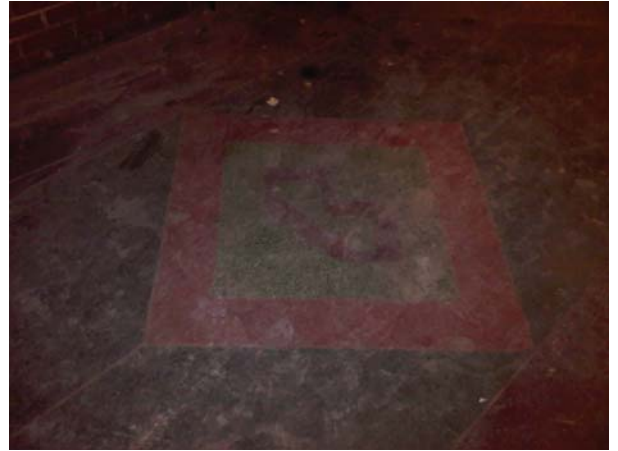
Photo 64 Detail view of terrazzo flooring w/ 'B' formed in centre of elevator lobbies
