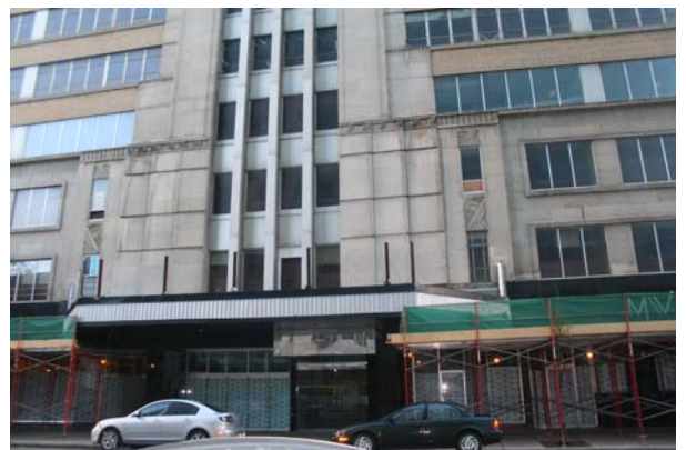
Photo 10 View of south entry façade & marquee remnants; scaffolding is in place as hoarding & to facilitate window replacement program
