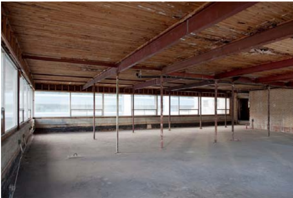
Photo 96 View of penthouse suite stripped down to bare structure w/ wood roof structural deck exposed
