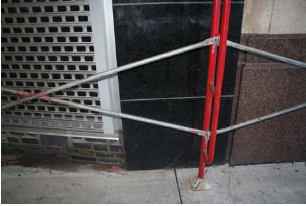
Photo 33 View of Rundle rock curb for storefront glazing adjacent to black granite pilaster at east end of south façade
