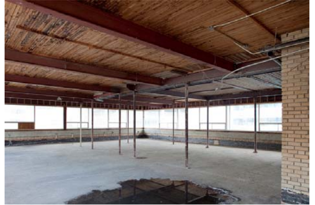
Photo 95 View of penthouse suite looking SE; roof of penthouse has been leaking for decades
