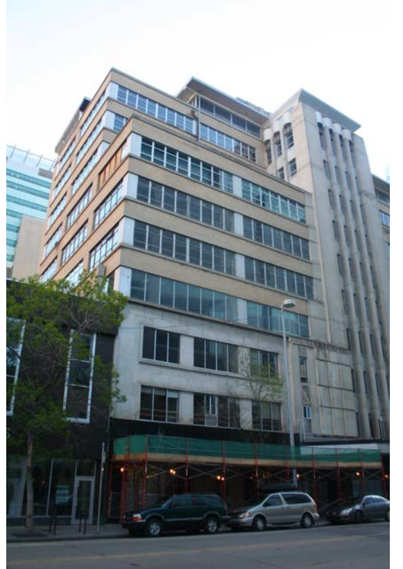
Photo 14 View of west wing & columnar frontispiece; scaffolding is in place to facilitate window replacement
