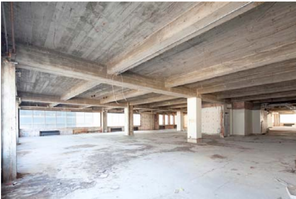
Photo 105 View looking NE toward elevator lobby from SW corner of 4 th to 7 th floors, typical
