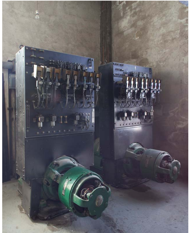
Photo 87 View of elevator controls & motors
