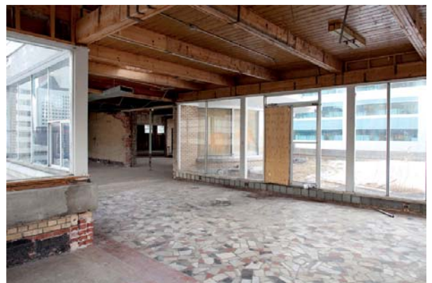
Photo 93 View of penthouse suite looking SE across patterned tile floor & out to exterior landscaped area on roof of 10 th floor below
