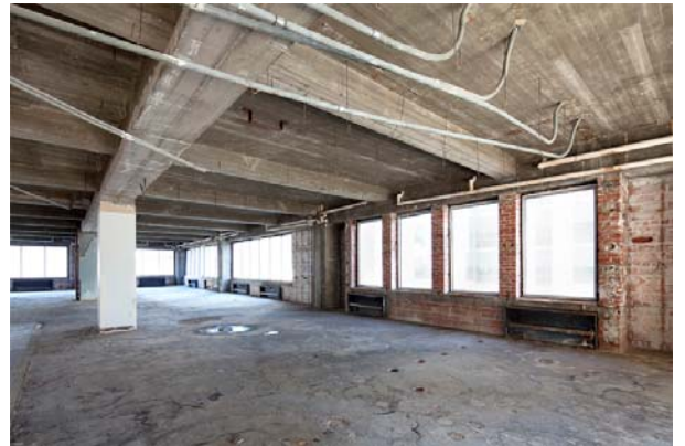
Photo 106 View looking SE from elevator lobby area to east wing of 4 th to 7 th floors, typical
