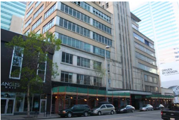
Photo 13 View of base & lower storeys looking NE; scaffolding is in place to facilitate window replacement
