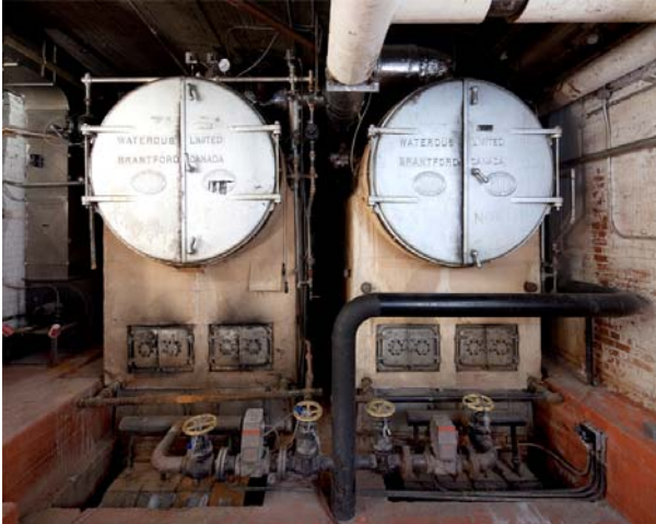
Photo 67 View of gas fired boilers for heating building & domestic hot water
