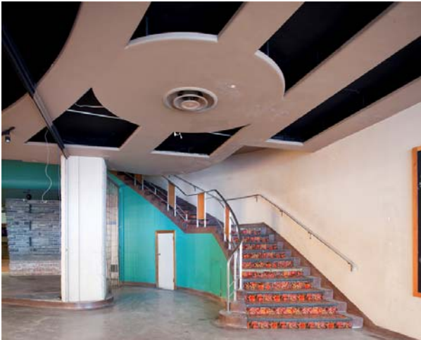
Photo 39 View of curved stair from theatre lobby to mezzanine level & theatre balcony; original ceiling infill panels have been removed
