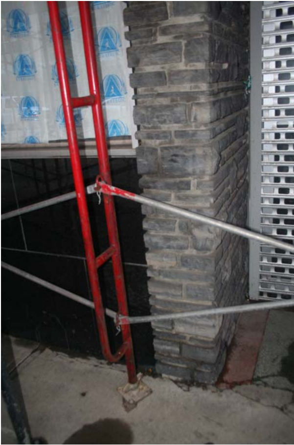
Photo 35 View of Rundle rock wing wall between black granite cladding & storefront entry; note the storefront entry with terrazzo flooring at the exterior; this condition is typical for exterior of theatre and office tower entries abutting city sidewalk
