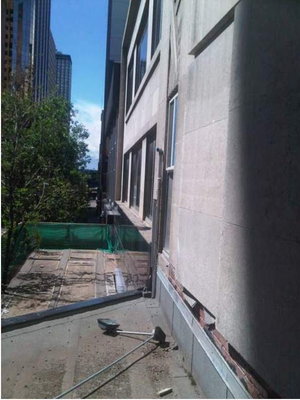
Photo 23 View on top of marquee looking west along Tyndall limestone & black granite beyond; scaffolding is in place to facilitate window replacement
