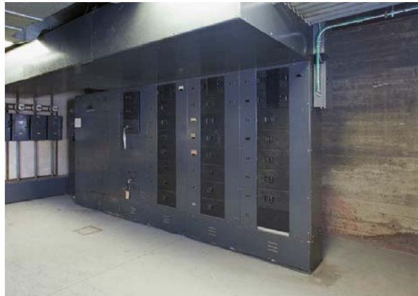
Photo 70 View of electrical panels
