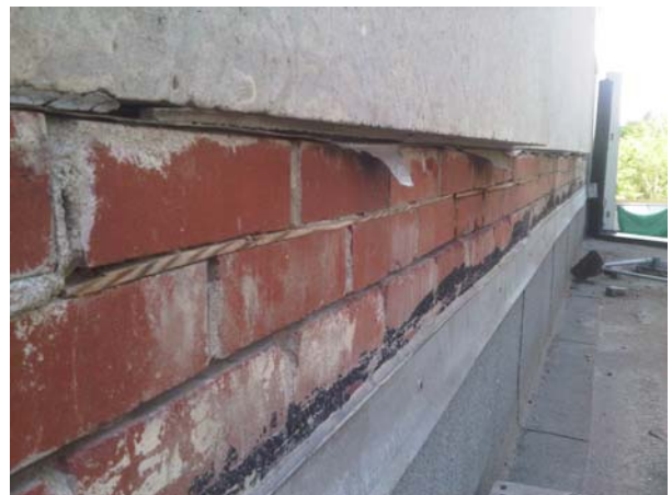
Photo 26 View of juncture of south wall & marquee; metal flashing embedded in brick mortar joint & tied into bituminous roofing membrane; cladding material removed limestone above and flashing below
