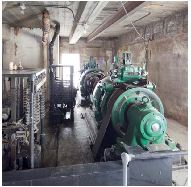
Photo 84 View of elevator machine room w/ motors
