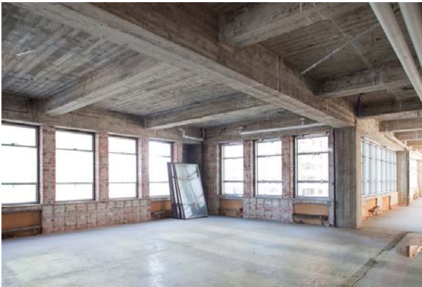
Photo 99 View of typical floor space in projecting area of columnar frontispiece on 8 th to 10 th floors looking SW
